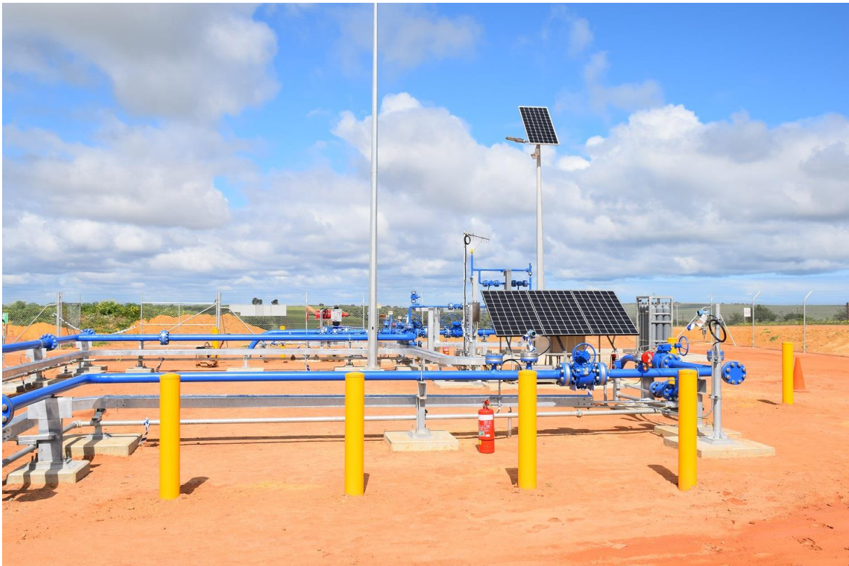
Figure 2-4 Indicative Hub (Existing Northern Hub constructed as part of Waitsia Stage 1 is shown)
