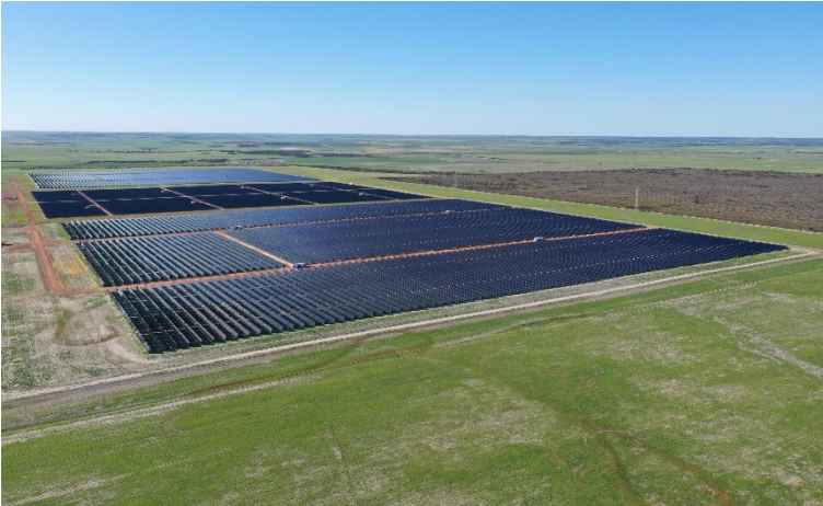
Figure 4: SynergyRED owned 40MW Greenough River Solar Farm
