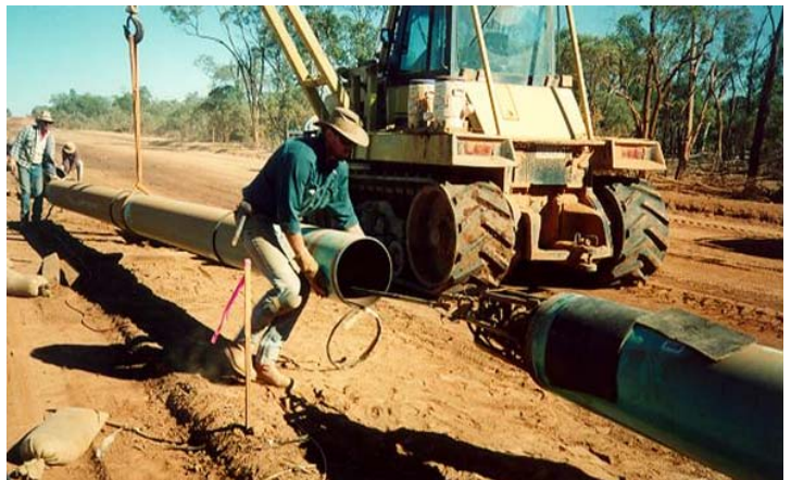
Figure 16 Epic Energy Pipeline
