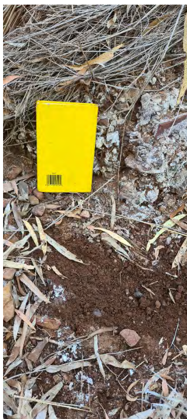
Plate 9: Salt Staining and potential lateral seepage (indicated by still damp alluvium)
