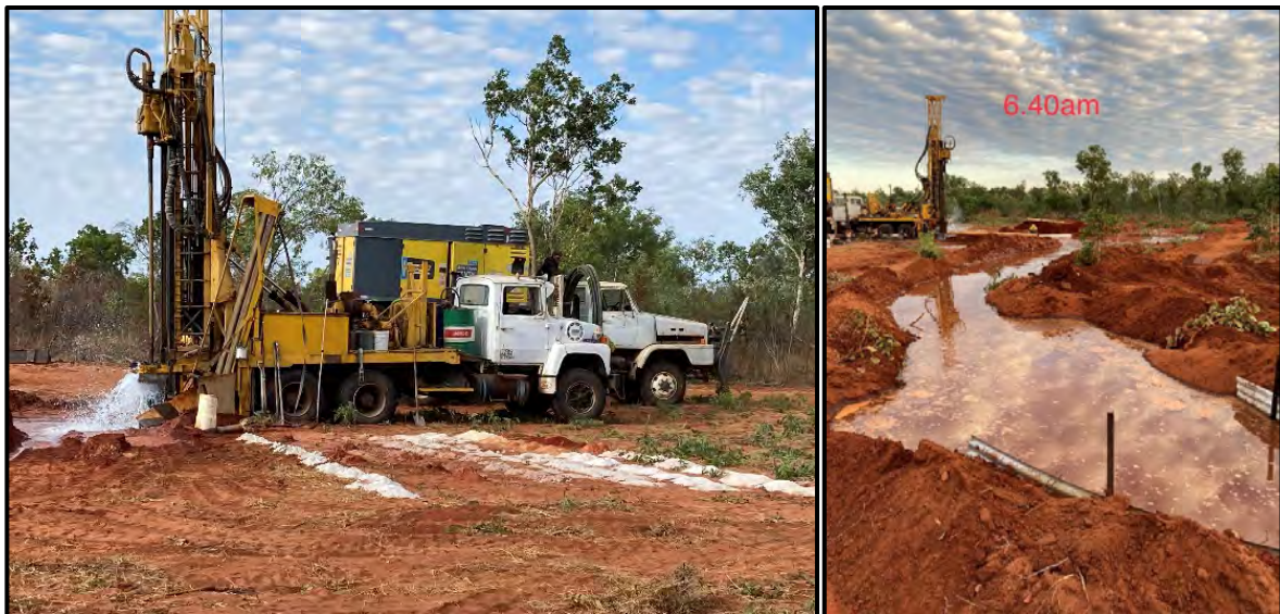
Figure 18. Drilling the test production bore at Scrubby site; note fine white sandstone in drill cuttings.
