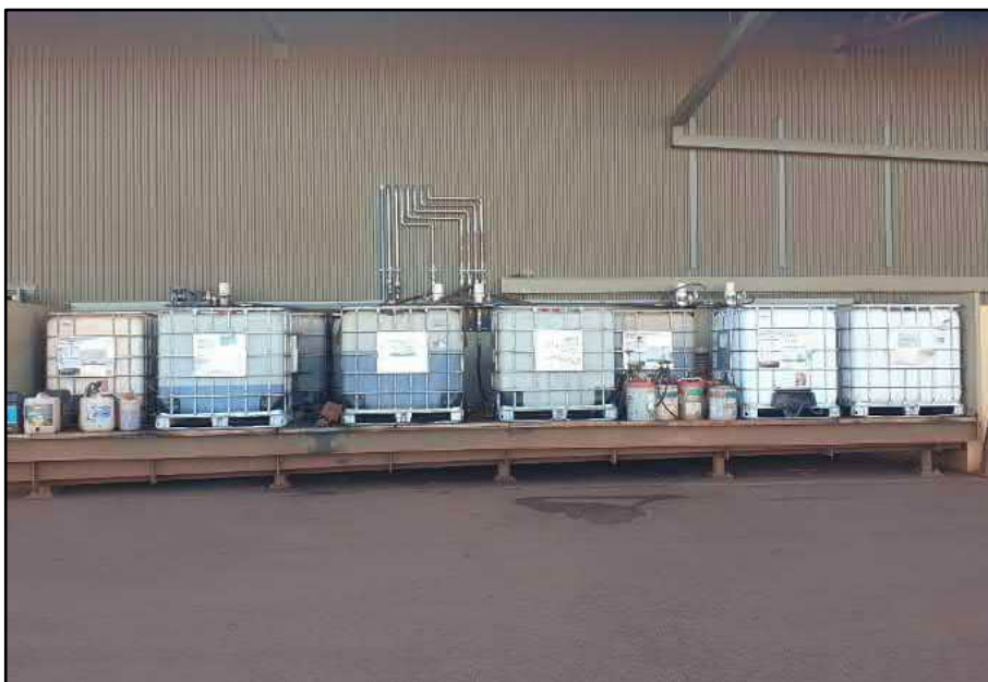
Photograph 2: Storage of chemicals in IBCs at the Infrastructure – OHP Maintenance Workshop. Chemicals include cleaning products, petroleum products such as oils and lubricants, and coolants
