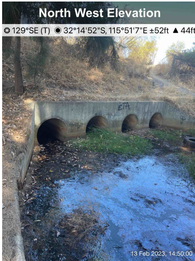
Photo 1. The exit of culvert of the Peel Sub O drain immediately west of the Freeway.
