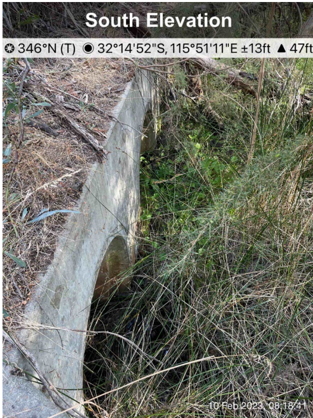
Photo 2. The inlet of the above culvert is obscured by vegetation immediately east of the Freeway.
