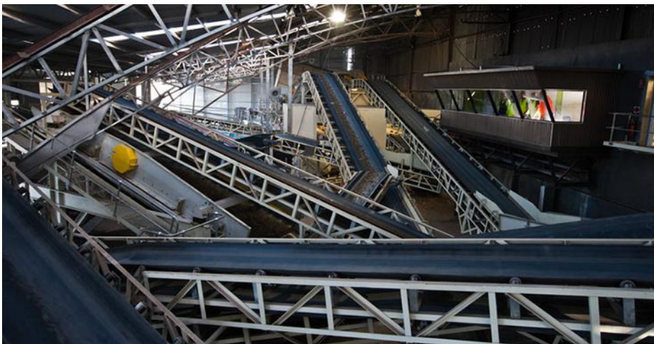
Figure 2: a network of conveyors, screeds and inspection points allows the mixed waste to be separated into individual streams.
