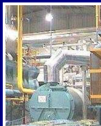
↑ Energy Utilization Heat Exchanger – steam boiler
