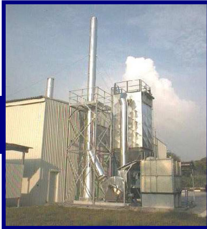
← Air Quality Control System
