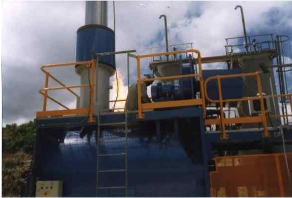
Figure 4: A leading US petroleum company operating in New Guinea installed an Entech Liquifire™ and PCG system to manage drill castings from oil and gas drilling.
