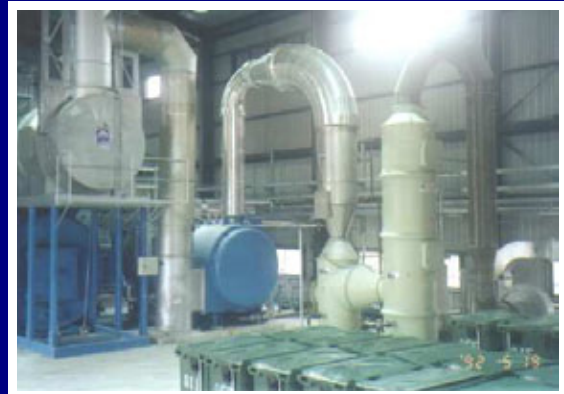
↑ Air Quality Control System (emissions are comparable to firing of natural gas).
