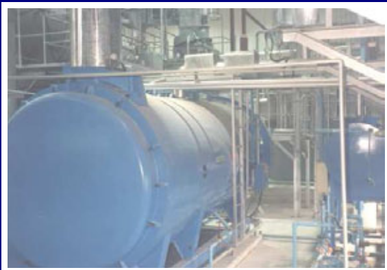
↑ Energy Utilization Heat Exchanger, where Syngas is fired.
