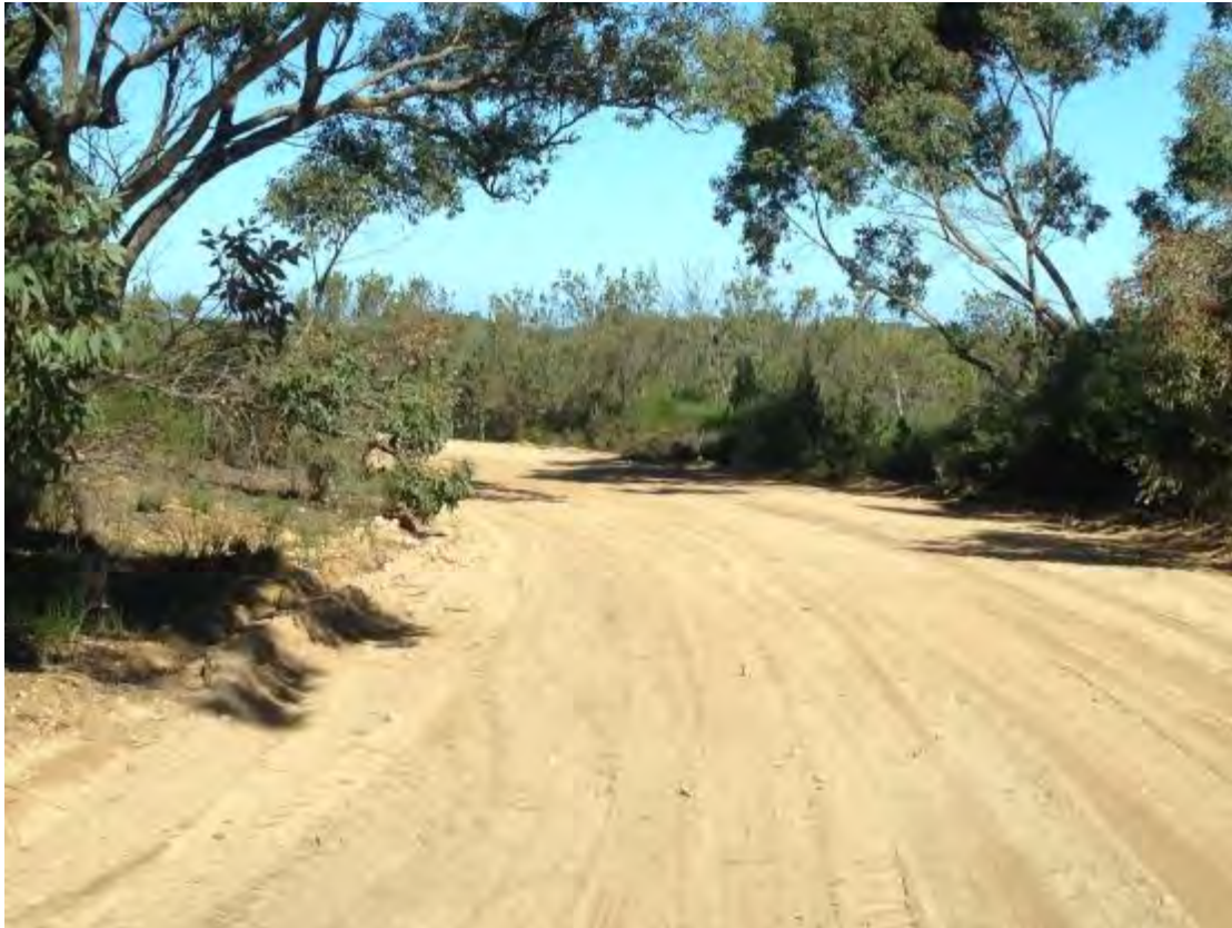
PBR North, SLK 3.9, vegetation overhanging road, obscuring sight distance
