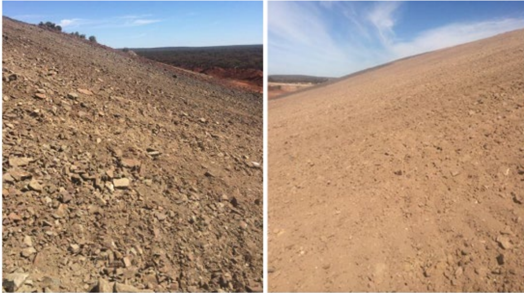
Figure 3: Example of an acceptable WRD surface batter free from flow converging features
