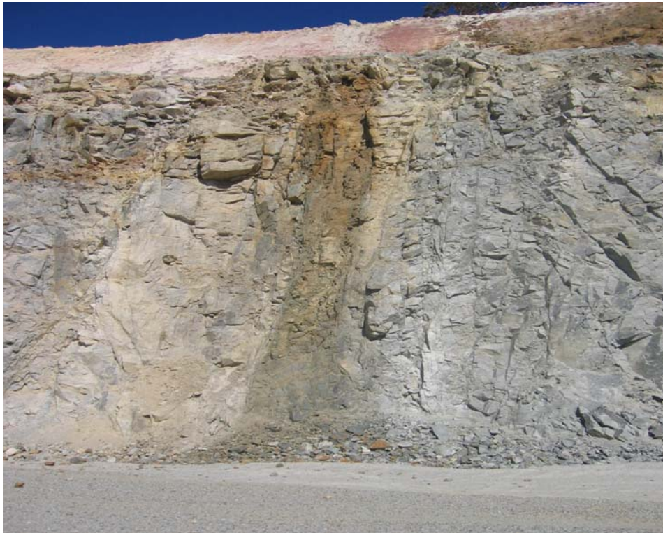
Plate 1: Fractures in granites in present quarry.
